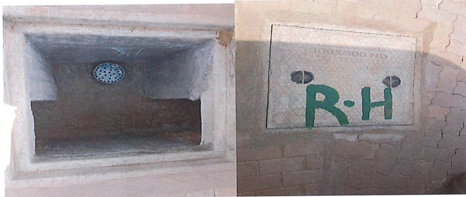
Rain water harvesting through the underground tanks
