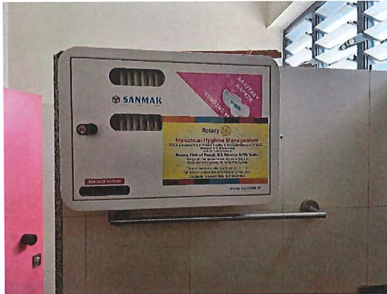
Installation of Sanitary Pad Dispenser in the women's washrooms
