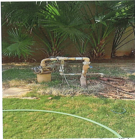
Bore Well Pump located at Vasant Rao Dempo Higher Secondary School of Science, Commerce and Arts
