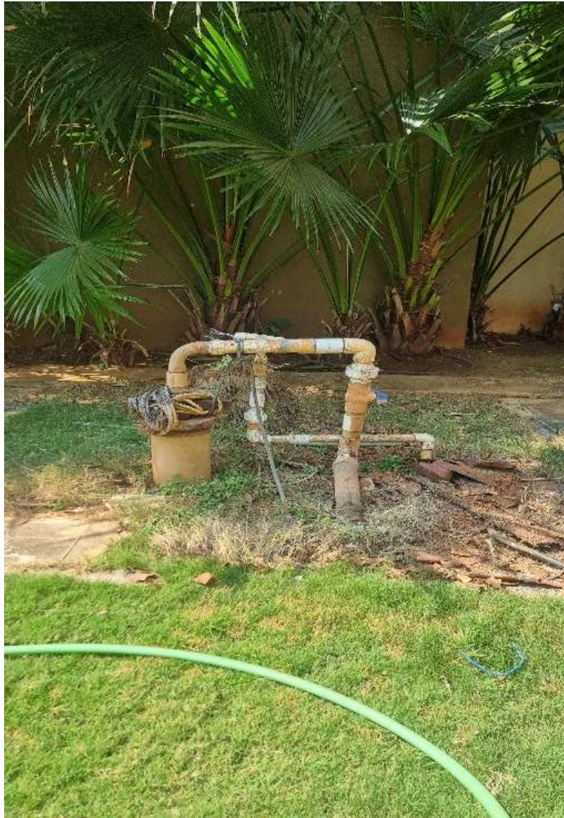
Figure 3 Bore Well Pump and Location
