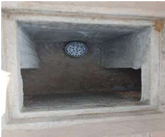
Figure 1 Rain Water Chambers for Water Storage
